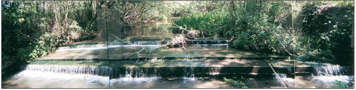
Figure 14. Fish Passage Barrier – Abandoned Dam Footings
