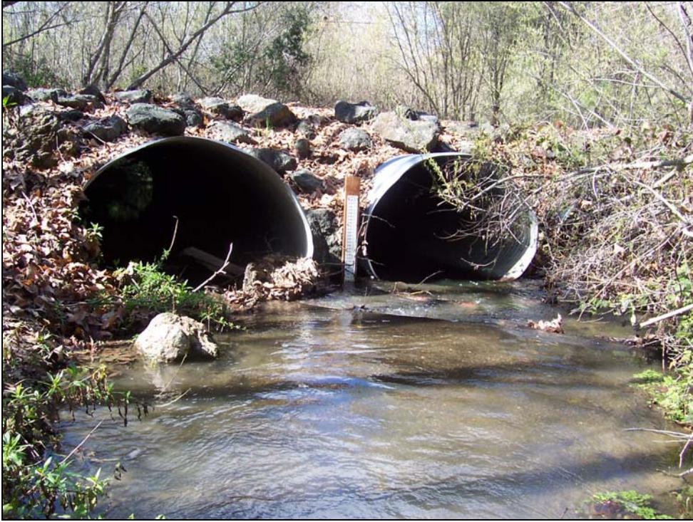
Figure 13. Fish Passage Barrier – Four Culverts at Biddle Park
