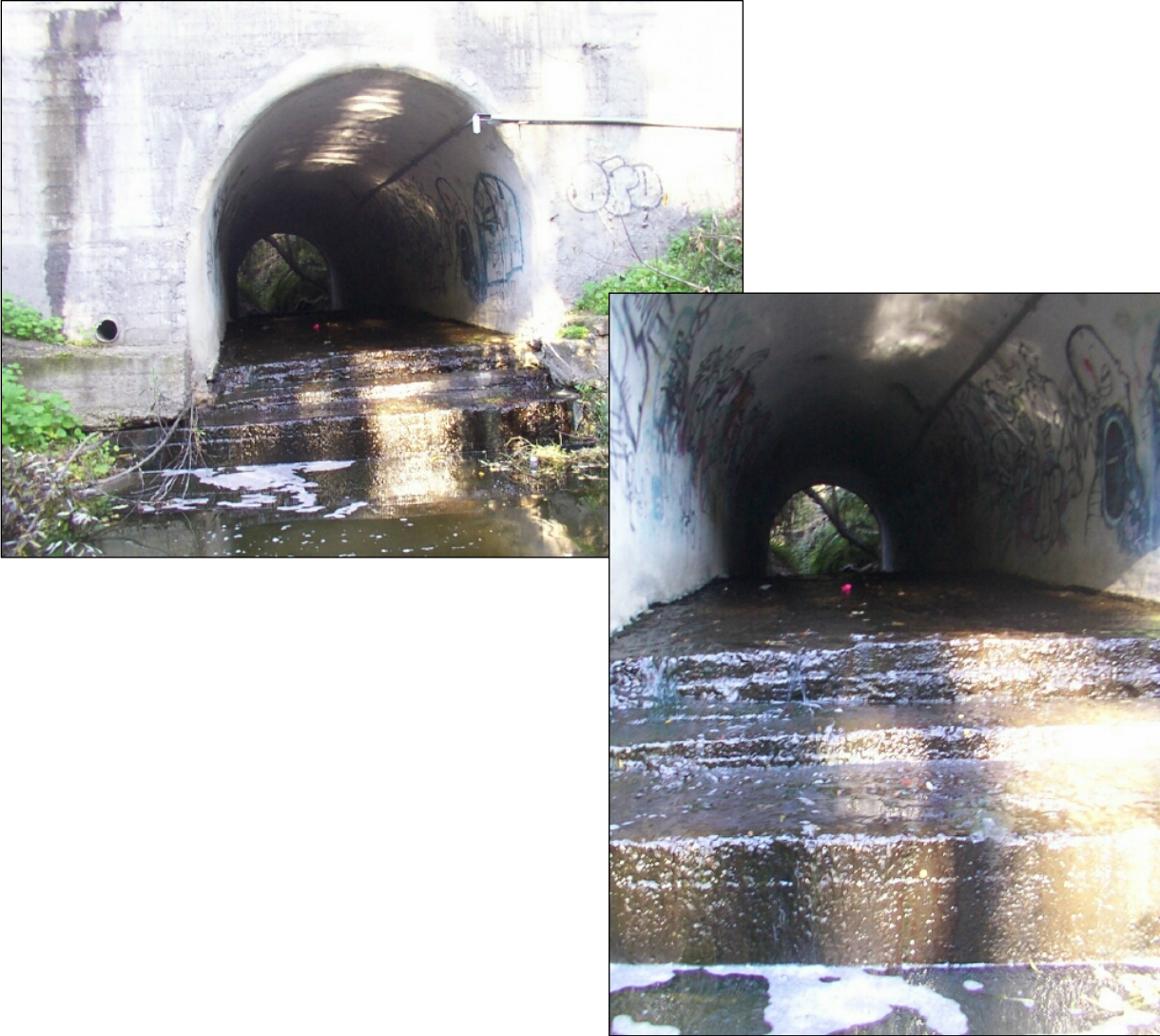
Figure 18. Fish Passage Barrier – Tally Ho Culvert
