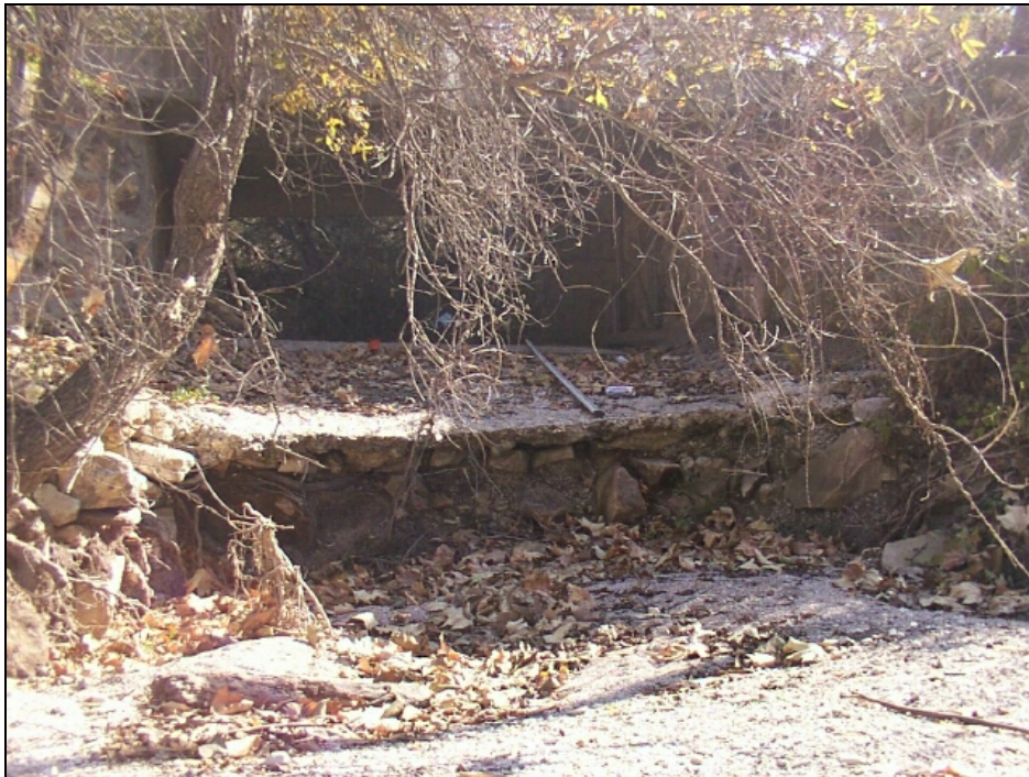
Figure 16. Fish Passage Barrier – Los Berros Creek Gauge
