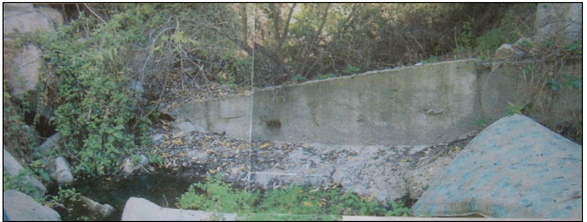
Figure 17. Fish Passage Barrier – Tar Springs Creek Concrete Weir
