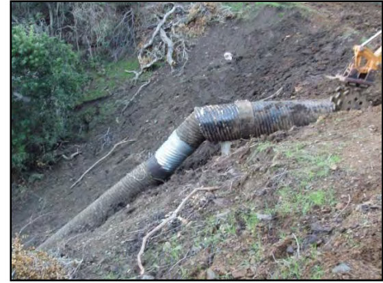
Figure 156. Extended downspout with new nipple.
