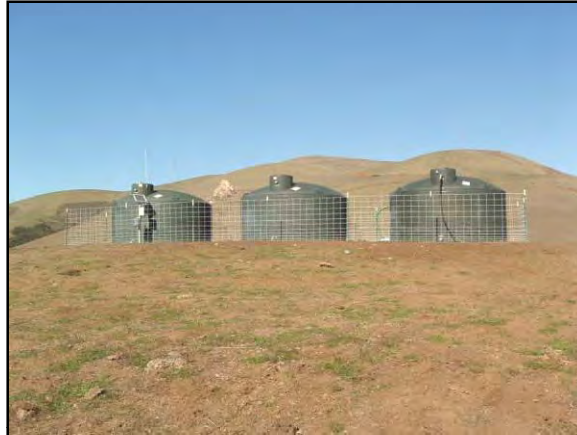
Figure 249. Three 4,500-gallon water tanks on north side of creek.
