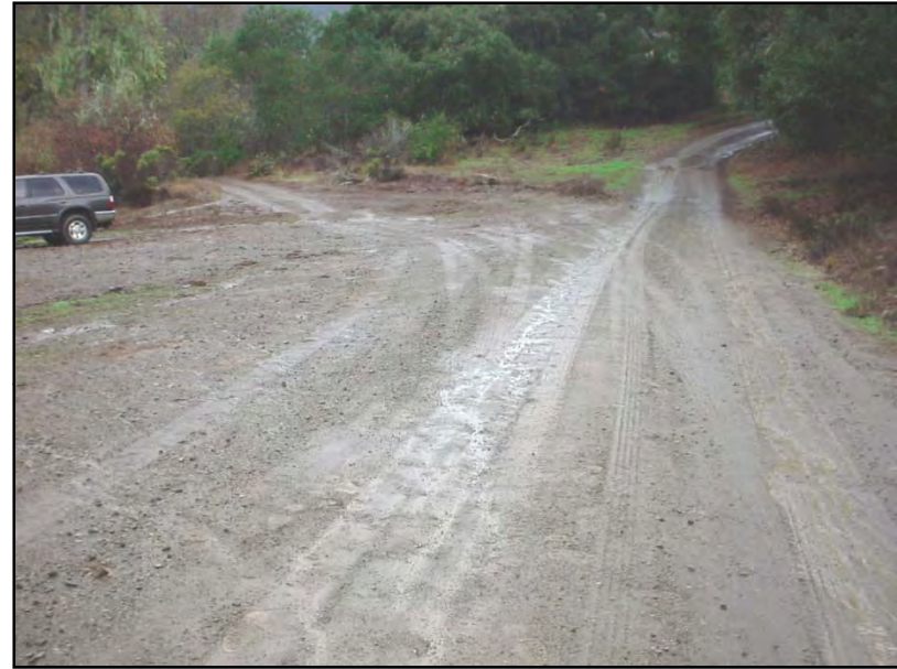
Figure 175. Road in need of repair.
