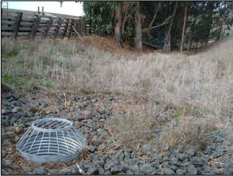
Figure 172. Looking upstream at drop structure and restored headcut, over a year after installation
