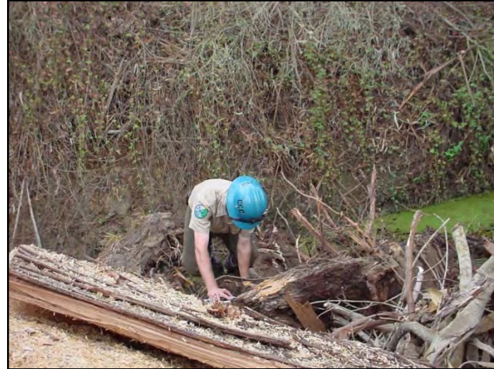
Figure 182. CCC crews chained trees and root wads so excavator could lift them out.
