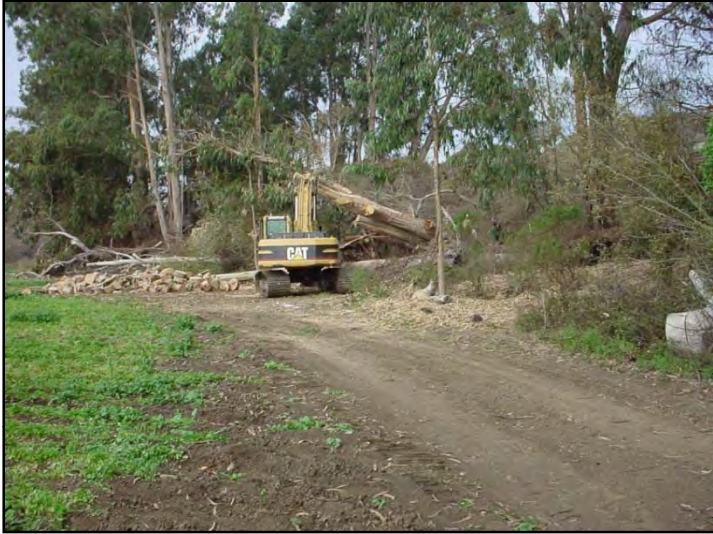
Figure 181. Excavator and operator lifting trees out with chain and bucket so as not to disturb banks.
