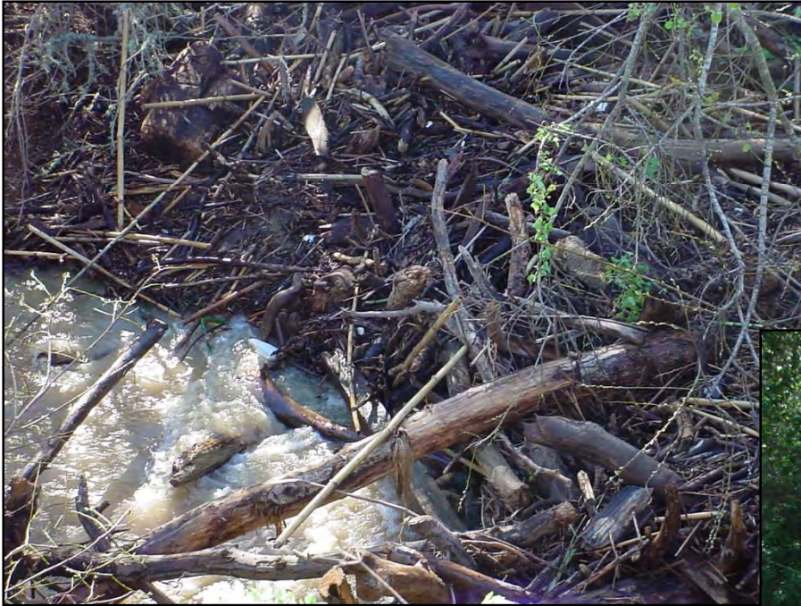
Figure 146. Substantial erosion due to debris jam.
