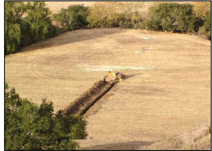
Figure 244. Backhoe used to install pipe in hayfield in order to get 48" depth.
