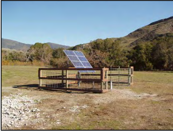
Figure 248. Solar panel and pump manifold at well site #2.
