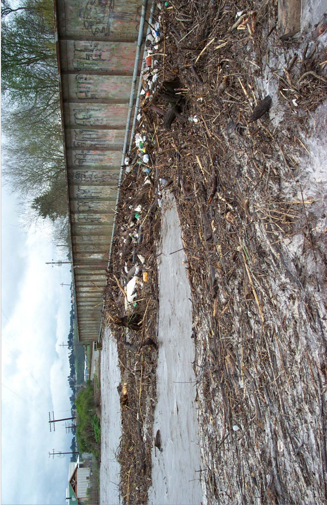
FIGURE 3.7: Debris and drift accumulation upstream of the Union Pacific Railroad Bridge during the March 2001 flood. This photo illustrates the need to modify, raise, or strengthen this bridge if an alternative that recommends levee raising is pursued (e.g. - Alternatives 3b and 3c). If the levees are raised without modifications to this bridge, water would inundate the bridge with the potential for failure.
