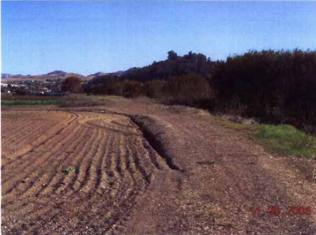
Photo 5: Low spot on north levee near approximate Station 103+50 –
