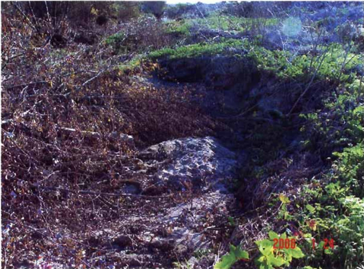
Photo 2: Scour around debris
