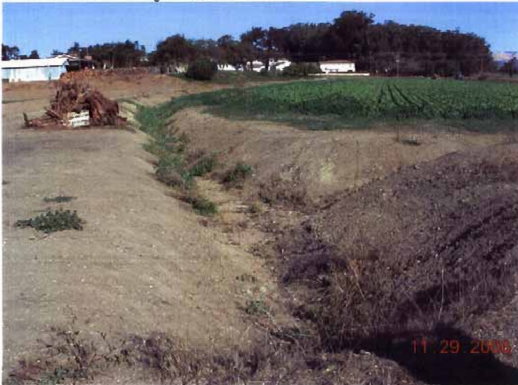
Photo 6: Earthen ditch contributing sediments to AG Creek –
