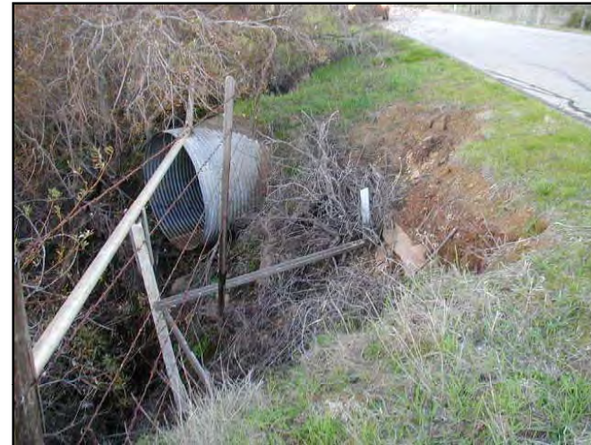
Figure 47. Source of head cut; 15 foot drop off.
