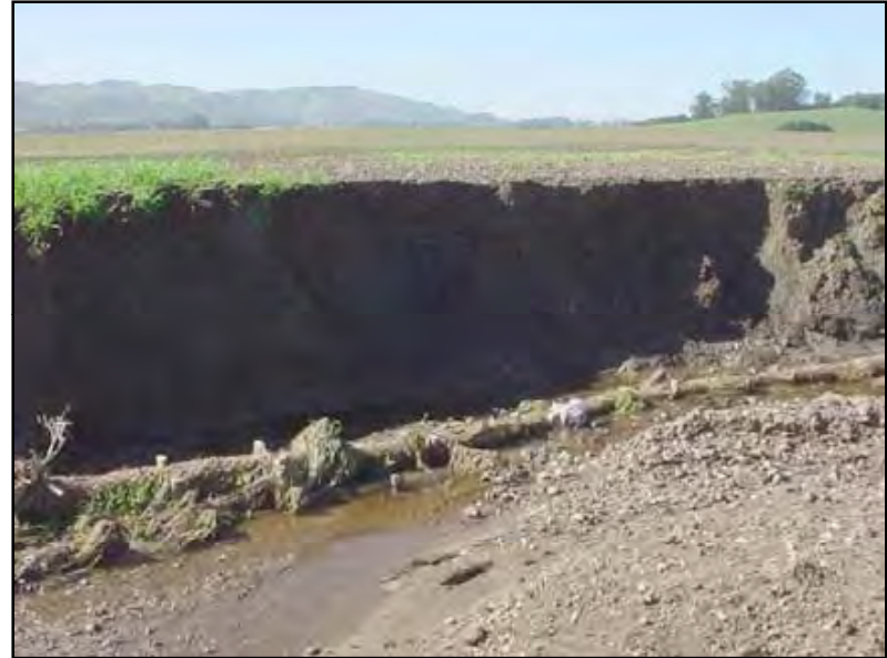
Figure 55. Bank erosion behind anchored coir logs.
