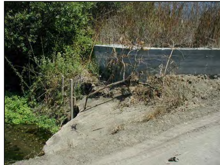
Figure 37. View of failing Arizona crossing.
