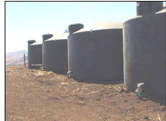
Figure 121. Four 5,000-gallon water tanks to supply 10 troughs.
