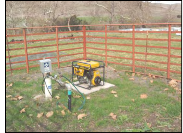
Figure 118. Well and generator.
