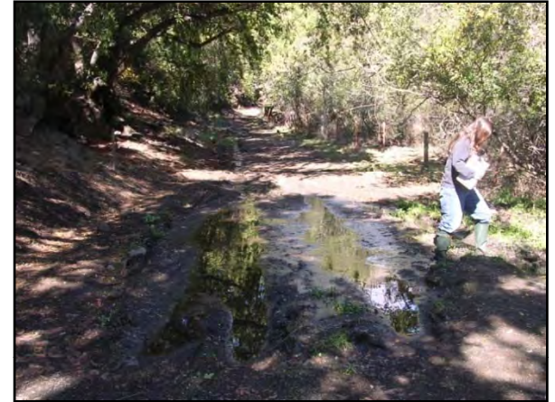
Figure 102. View of a seep in the road.
