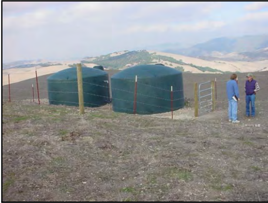
Figure 93. Installed water tanks.
