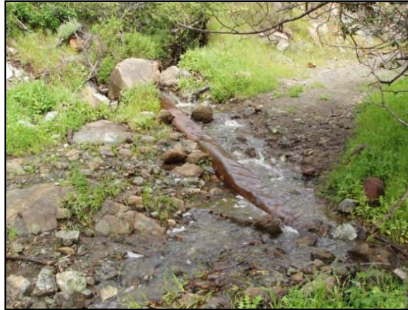
Figure 101. Failed culvert was replaced
