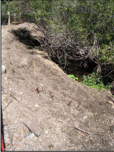
Figure 100. Sloughing bank due to seep.
