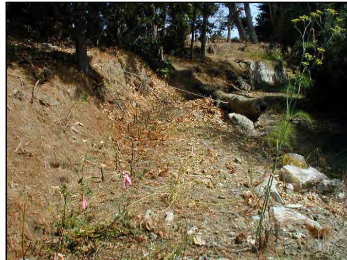
Figure 12. Note cable securing log.
