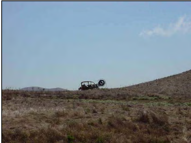
Figure 114. Distant view of cat ripping in pipe – note spool of pipe on right side of cat.
