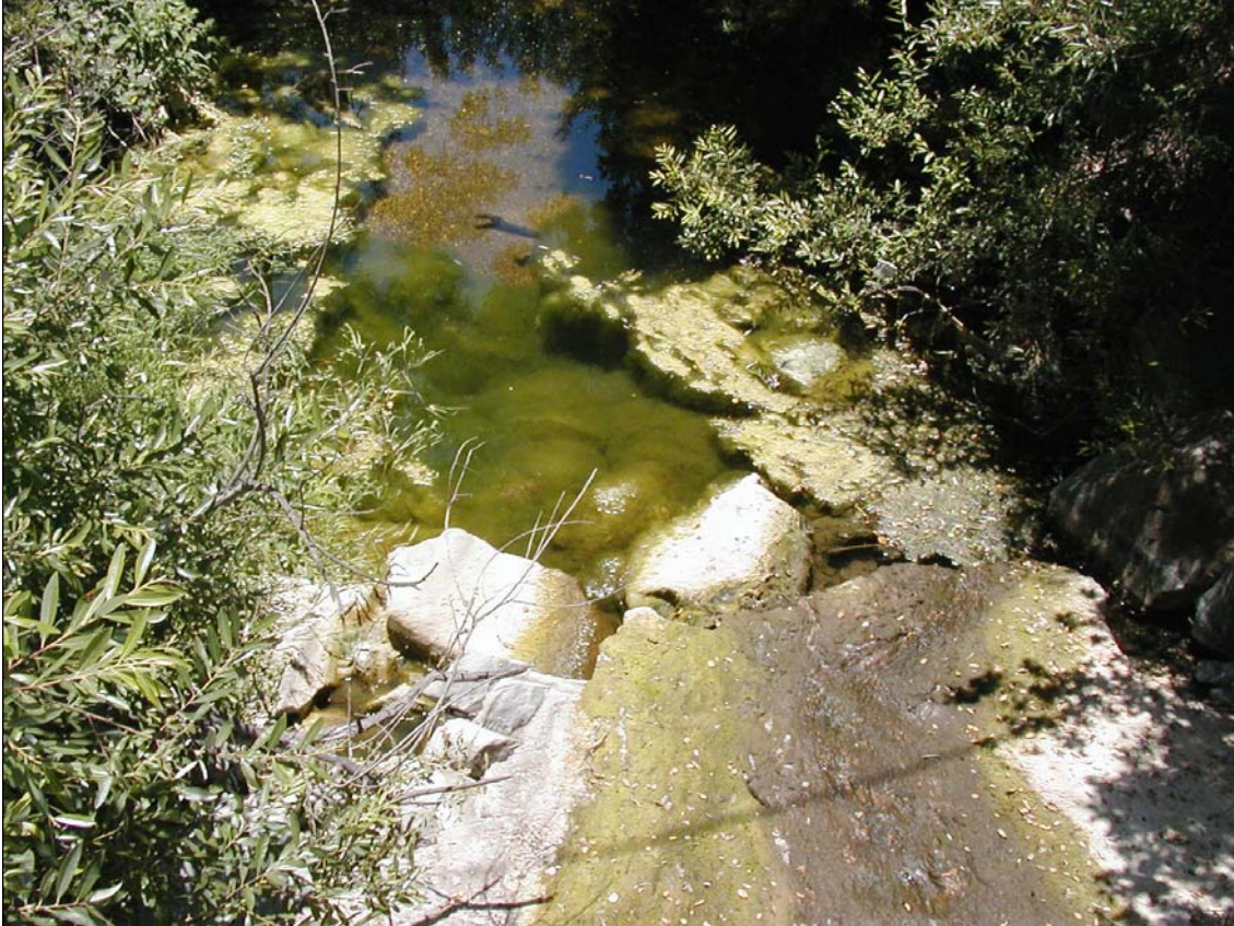
FIGURE 3.6 WEST CORRAL DE PIEDRA CREEK FISH BARRIER AT COUNTY BRIDGE ON RIGHETTI ROAD
